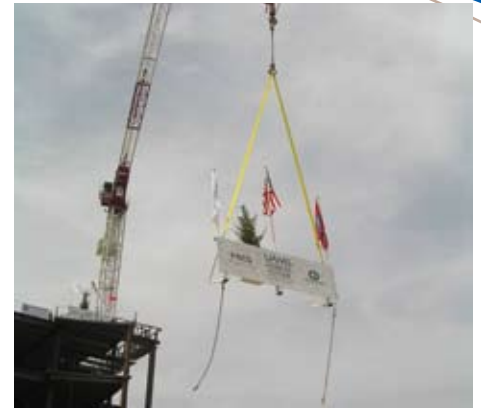
The final beam is raised for placement at the top of the PRI.
